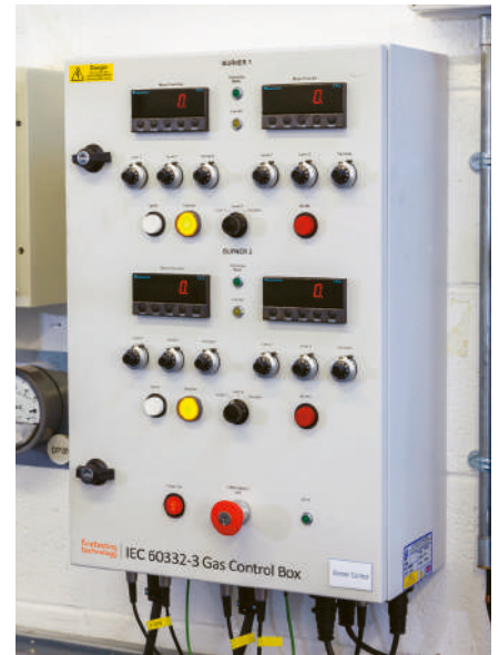
Gas control box mounted on wall
